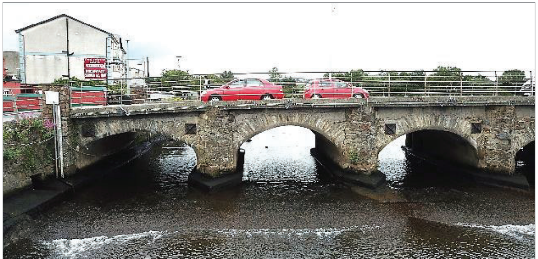
Typical arch detail showing concrete downstream apron and pattress plates and also just visible spray concrete to underside of arches. Photo c/o Brady Shipman
