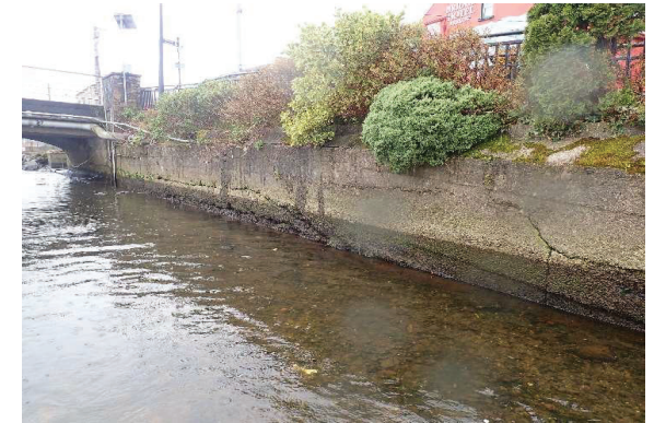
South Bank - west, upstream side. This bank will be altered as part of the process of inserting new Main sewer.
