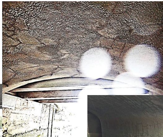
Underside of arch concrete sprayed - possible during the masonry works in 1982 or the later the Larson works of 2013, now crazing. All loose and crazed render should be removed to allow close inspection of original fabric and repair by re-packing all empty, leached out mortar joints.
