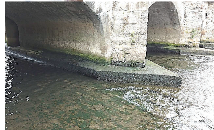
Typical downstream detail - significant erosion of pointing from breakwater masonry above concrete apron. This will require re-pointing and re-seating of any loose stones work. Repoint and repair will also allow for a clean up of gunite overspray and give an enhanced visual of the historic masonry.
