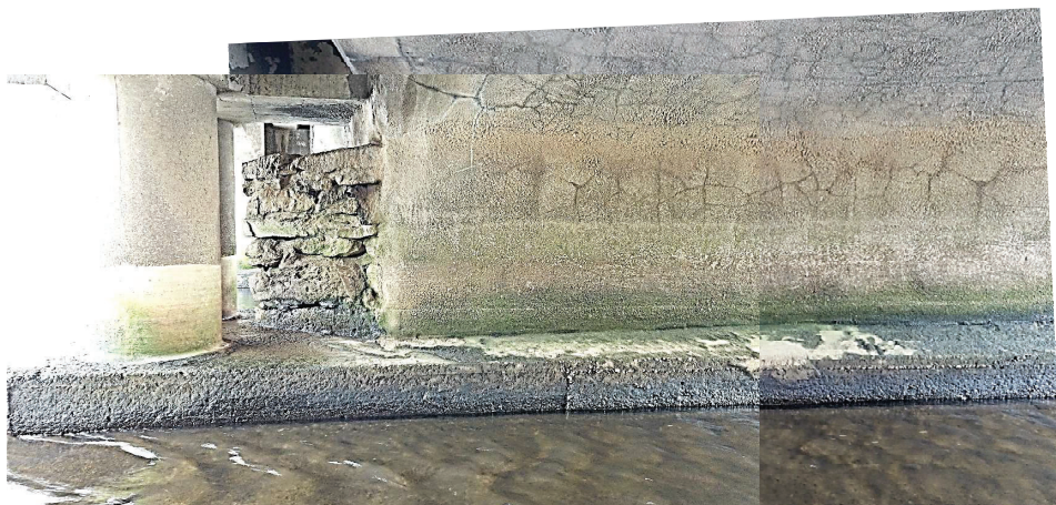
Typical upstream detail of historic bridge under canopy of newer section - significant erosion of pointing from breakwater. This will require re-pointing and re-seating of any loose stonework.
