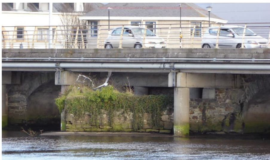
Central pier of historic bridge over sailed by later bridge. Photo c/o CourtneyDeery
